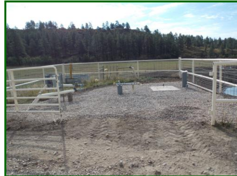
High production water well
