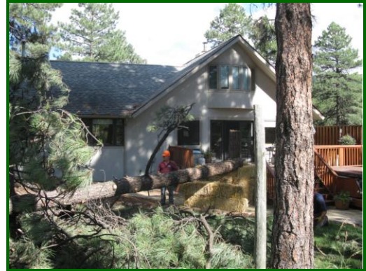
Cutting down a large ponderosa pine that was growing up through the deck at a home in Florida River Estates.
