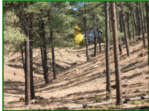
Mitigation work on a slope below a home in Deer Valley Estates.
