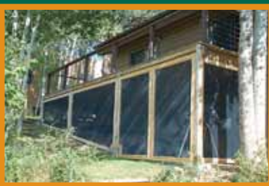
Figure 16: Enclosing decks with metal screens can prevent embers from igniting a house. Photo: Marilyn Brown, La Plata County
