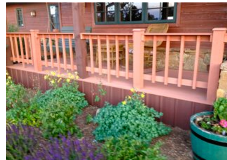
Enclosing the area below the deck with corrugated metal, propanel, or other screening will reduce a structure’s vulnerability to flying embers, the most common home ignition problem.
