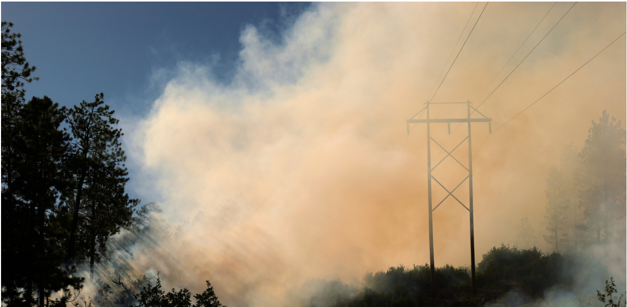
Reducing fuel loading under and around the Tri-State transmission lines was a central focus during Dry Lake
